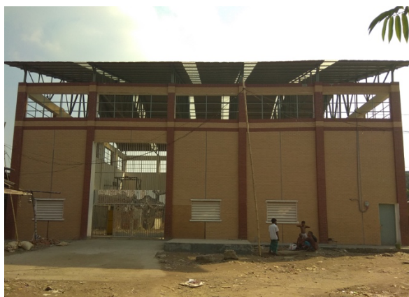
Waste transfer station, DSCC
