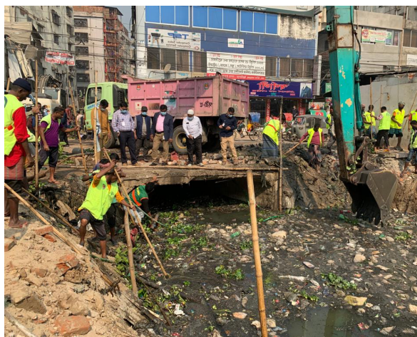
Drain cleaning program
